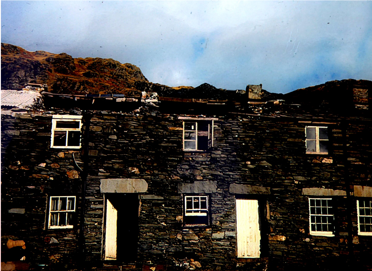
Two photos of the cottage in its initial delapidated state.
